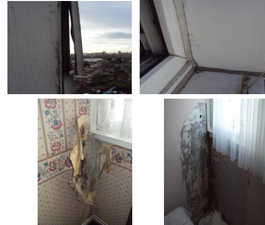
Fig 3. Dampness issues in flats A (right) and B (left)
